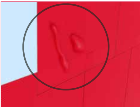
Fig.03: 'Bubbles' caused by insufficient pressure when installing Wraptite.
